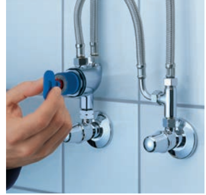
2. Technical disinfection without new calibration
